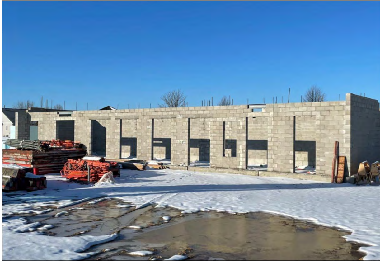
Masonry at Fire Unit Turn-Out Gear
